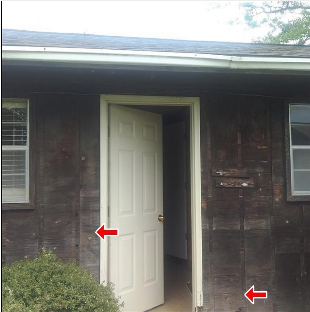
2.0 Item 2(Picture) Exterior wall siding, trim, and fascia on Cottage needs to be painted or stained to prevent wood rot.
