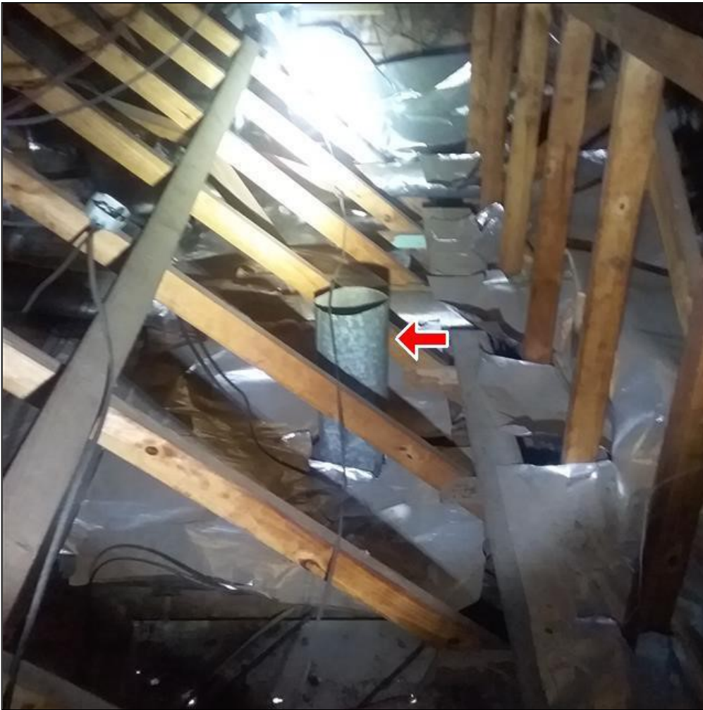
9.4 Item 1(Picture) Kitchen exhaust Hood pipe needs to be vented through roof to exterior.
