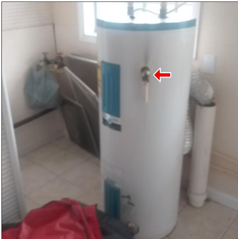
6.2 Item 1(Picture) Cottage water heater needs to have pressure / temperature relief valve piped to exterior.
