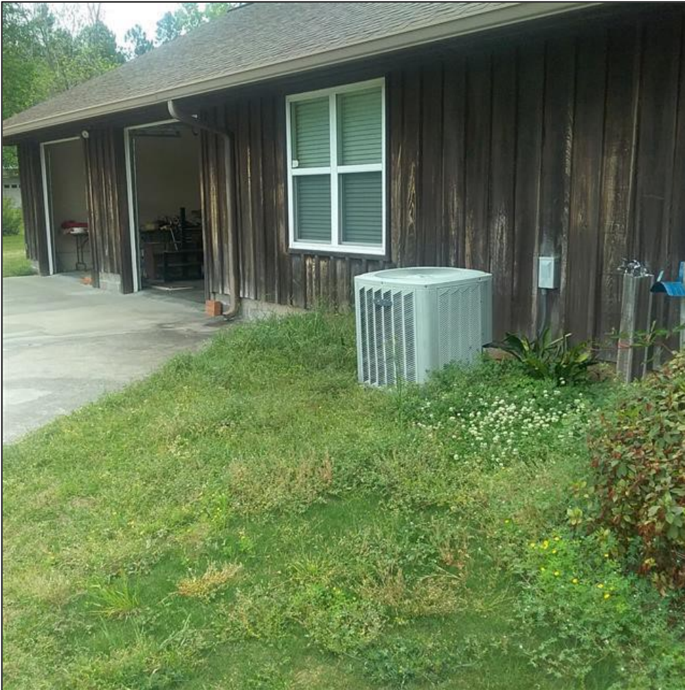
8.8 Item 2(Picture) The HVAC system serving the middle portion of home is at end of its expected service life, and will need to be replaced in the near future.
