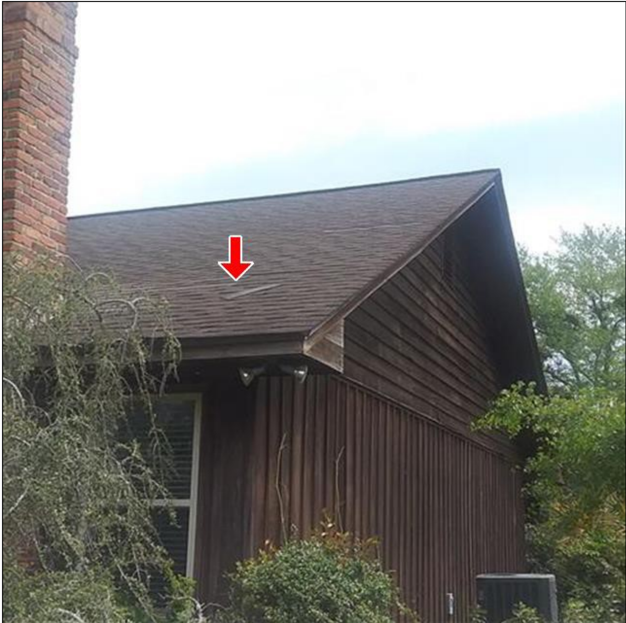
1.0 Item 1(Picture) The roofing has a shingle loose to the right side of home. (2) Cottage roof gutter needs to be straightened or replaced.
