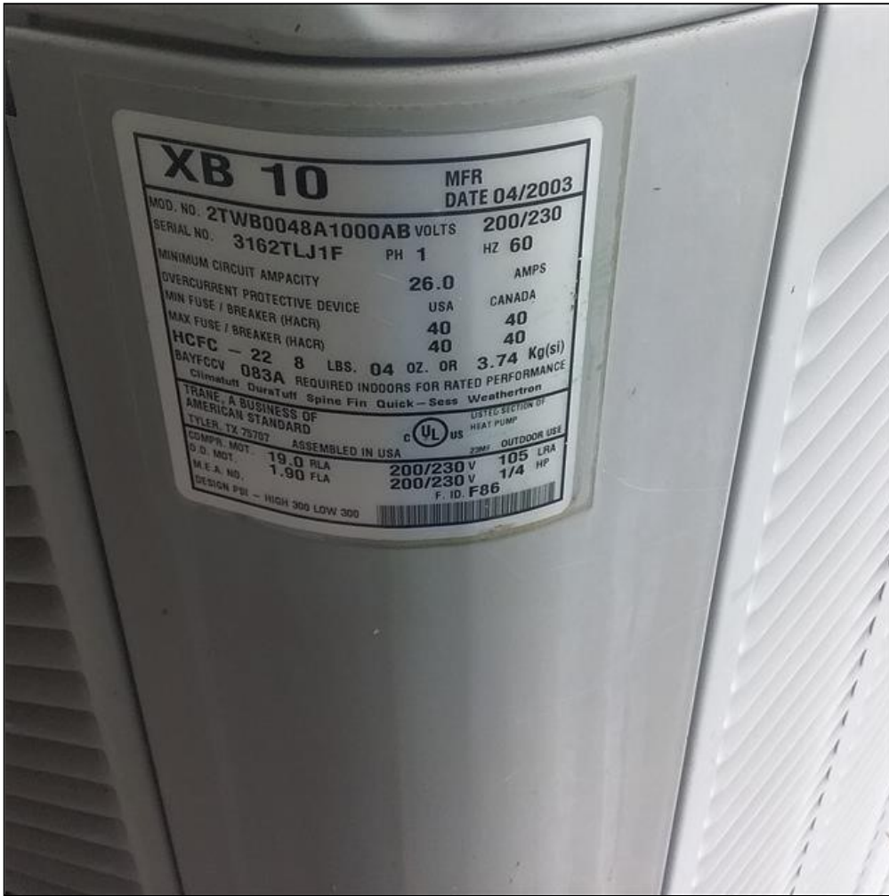
8.8 Item 3(Picture) The HVAC system serving the middle portion of home is at end of its expected service life, and will need to be replaced in the near future.
