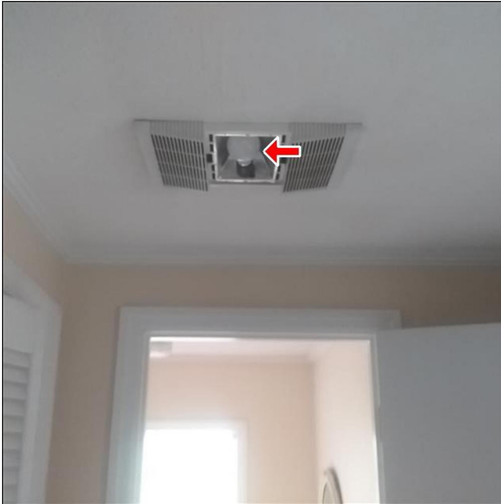
7.3 Item 3(Picture) Light needs cover in bathroom.
