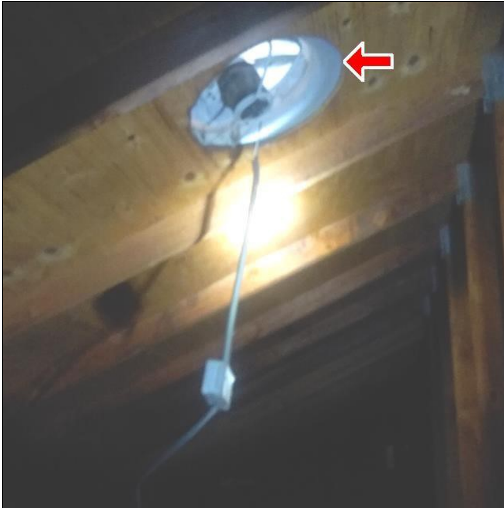
9.5 Item 1(Picture) Both roof attic power ventilator motors are bad, and need to be replaced.
