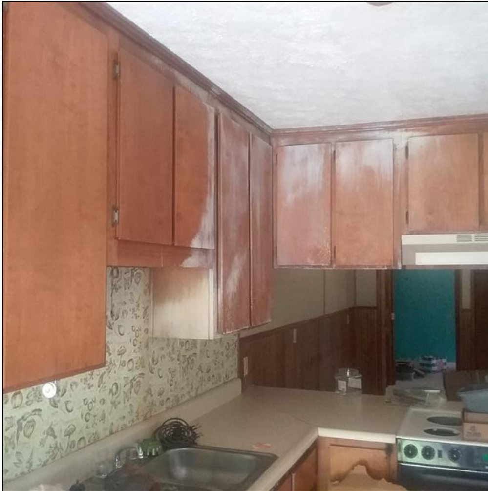
4.4 Item 1(Picture) Cottage cabinets need to be cleaned, and re-stained.
