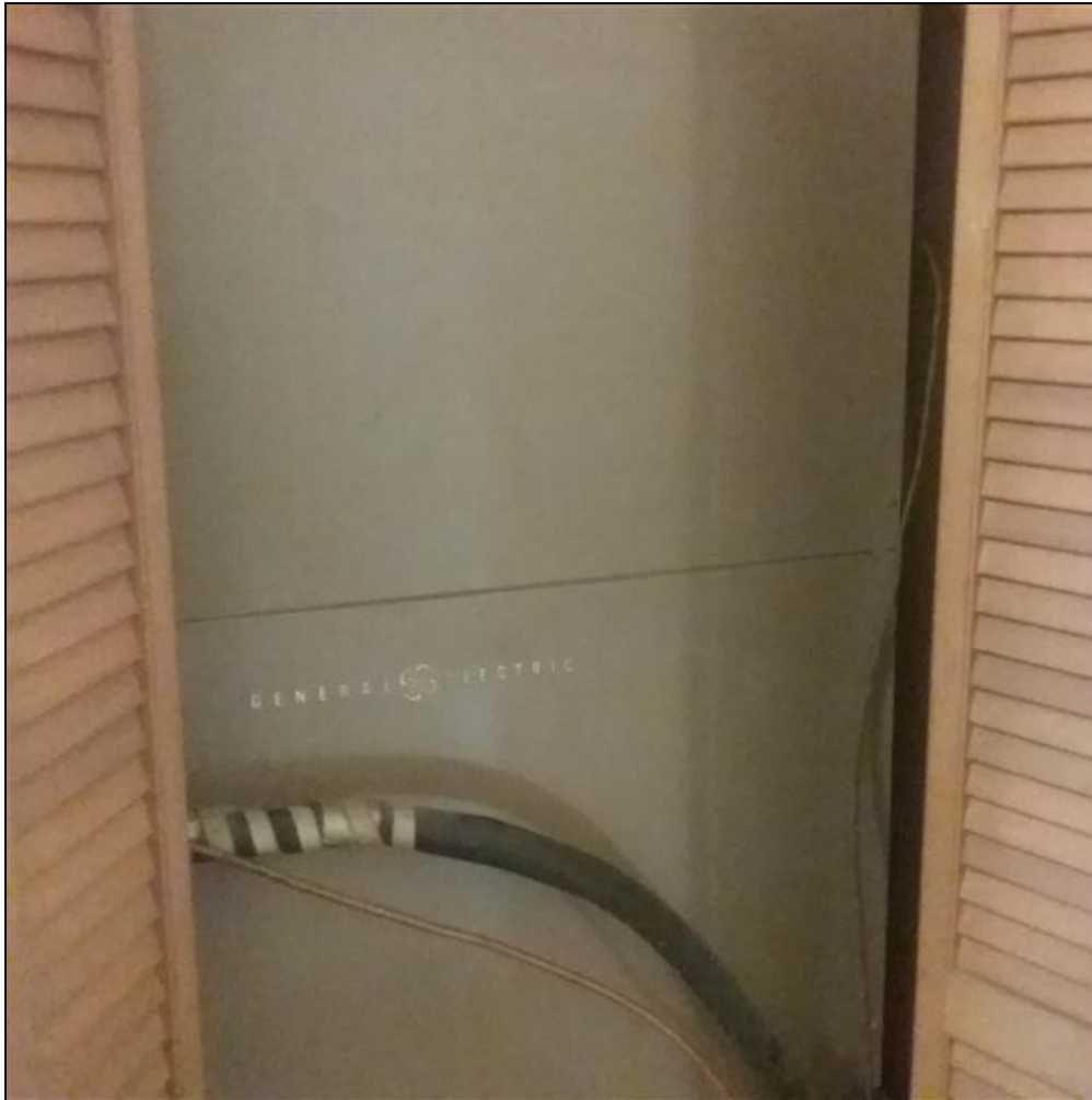
8.8 Item 4(Picture) The HVAC system serving the middle portion of home is at end of its expected service life, and will need to be replaced in the near future.
