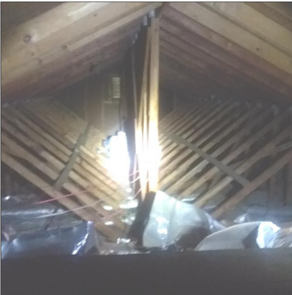
9.0 Item 2(Picture) Attic could use more insulation. Current insulation is around R-25.
