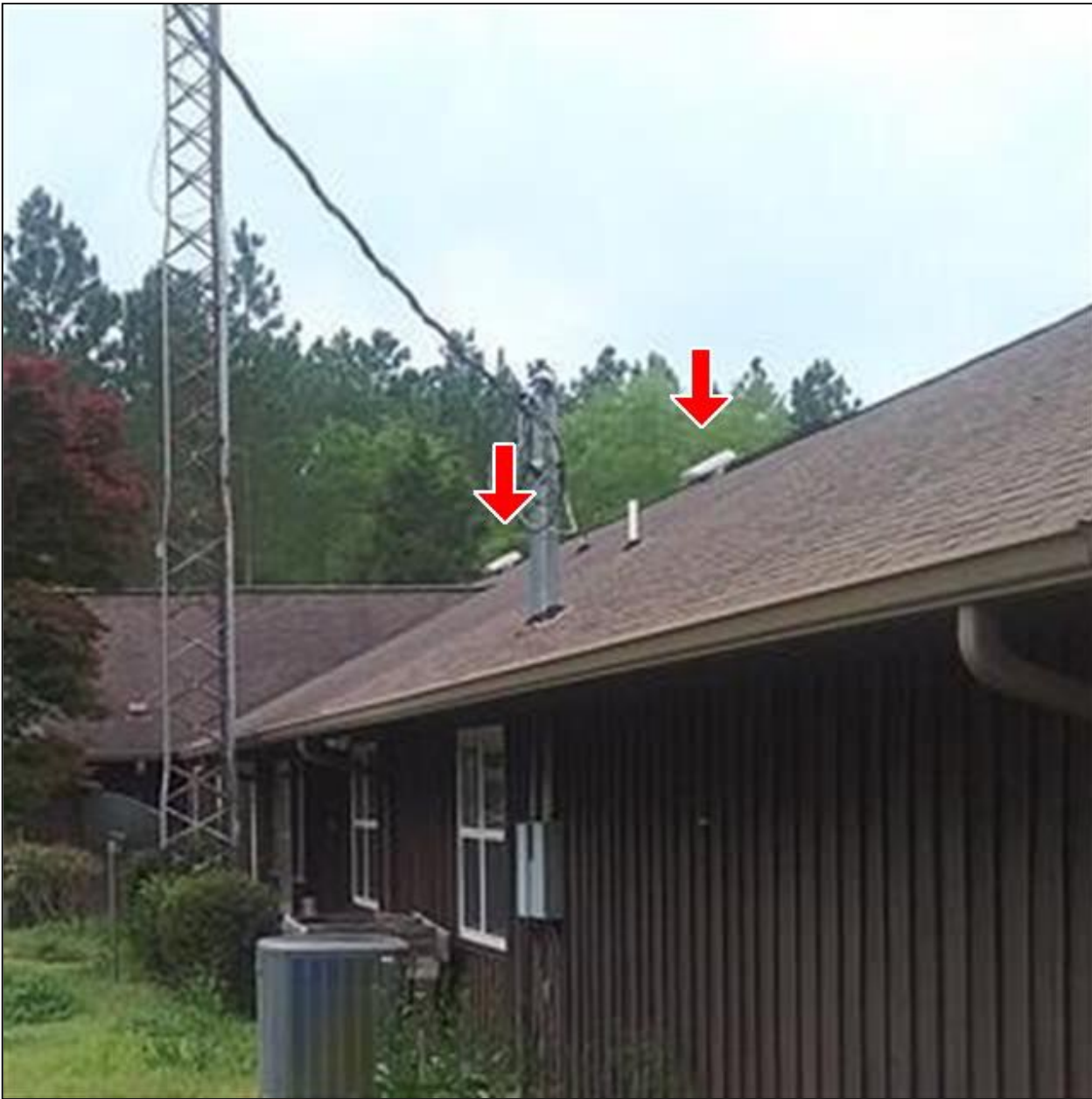
9.5 Item 2(Picture) Both roof attic power ventilator motors are bad, and need to be replaced.
