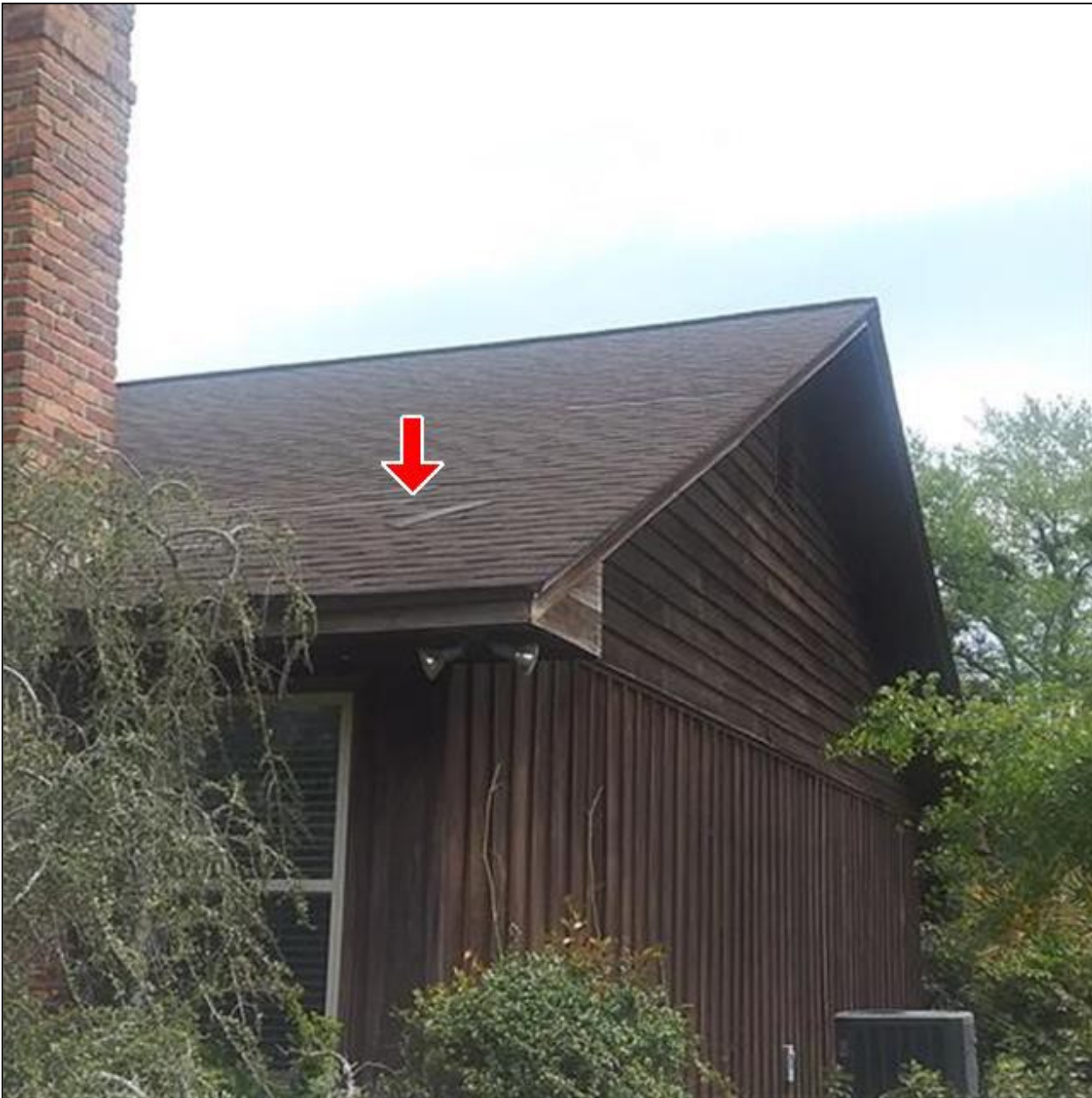
1.0 Item 1(Picture) The roofing has a shingle loose to the right side of home.
