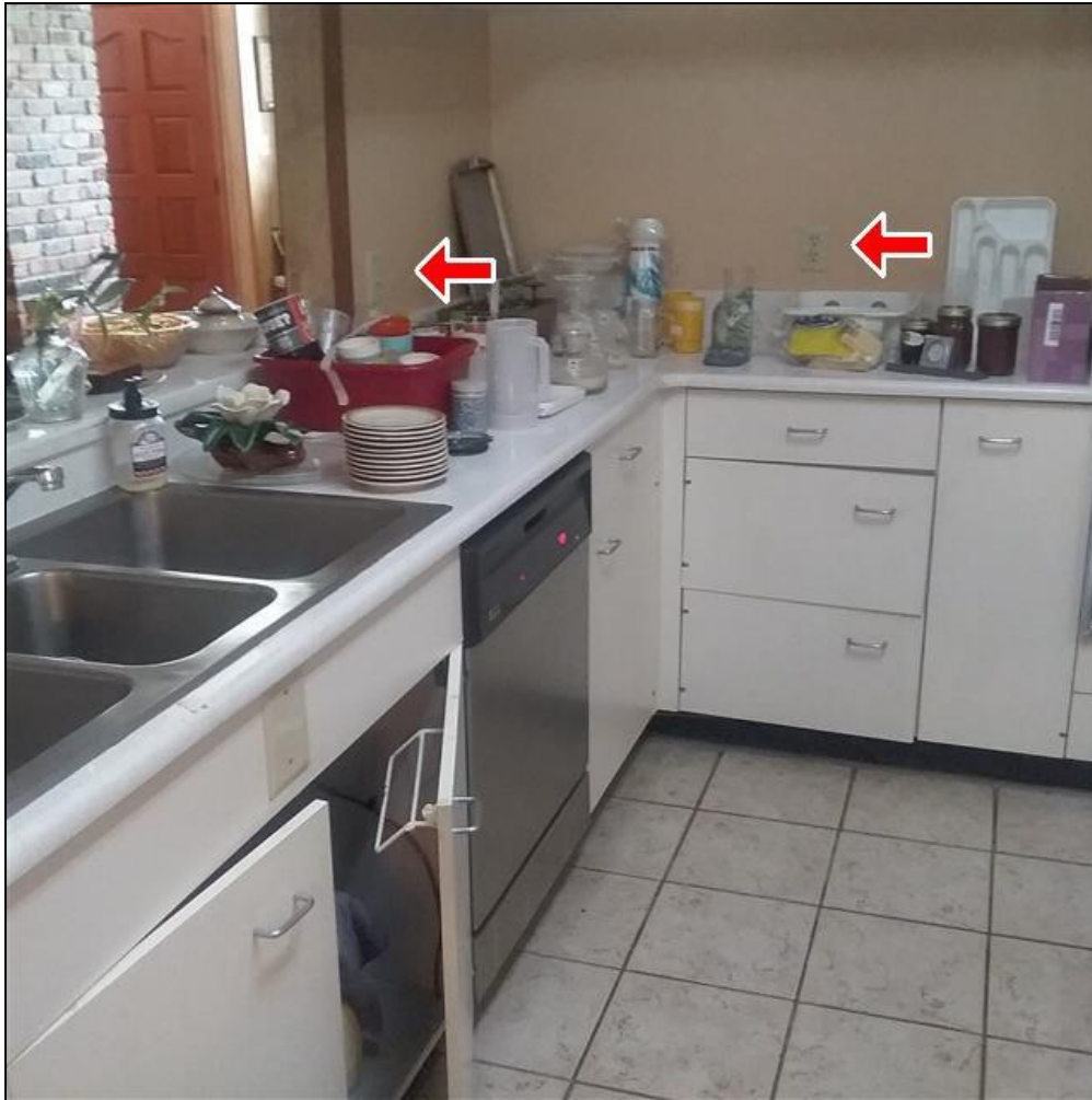
7.5 Item 6(Picture) Receptacle needs to be changed to GFCI type receptacle.
