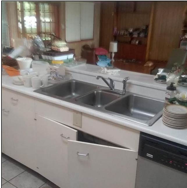
6.1 Item 1(Picture) The hot water side of kitchen faucet did not function when tested.
