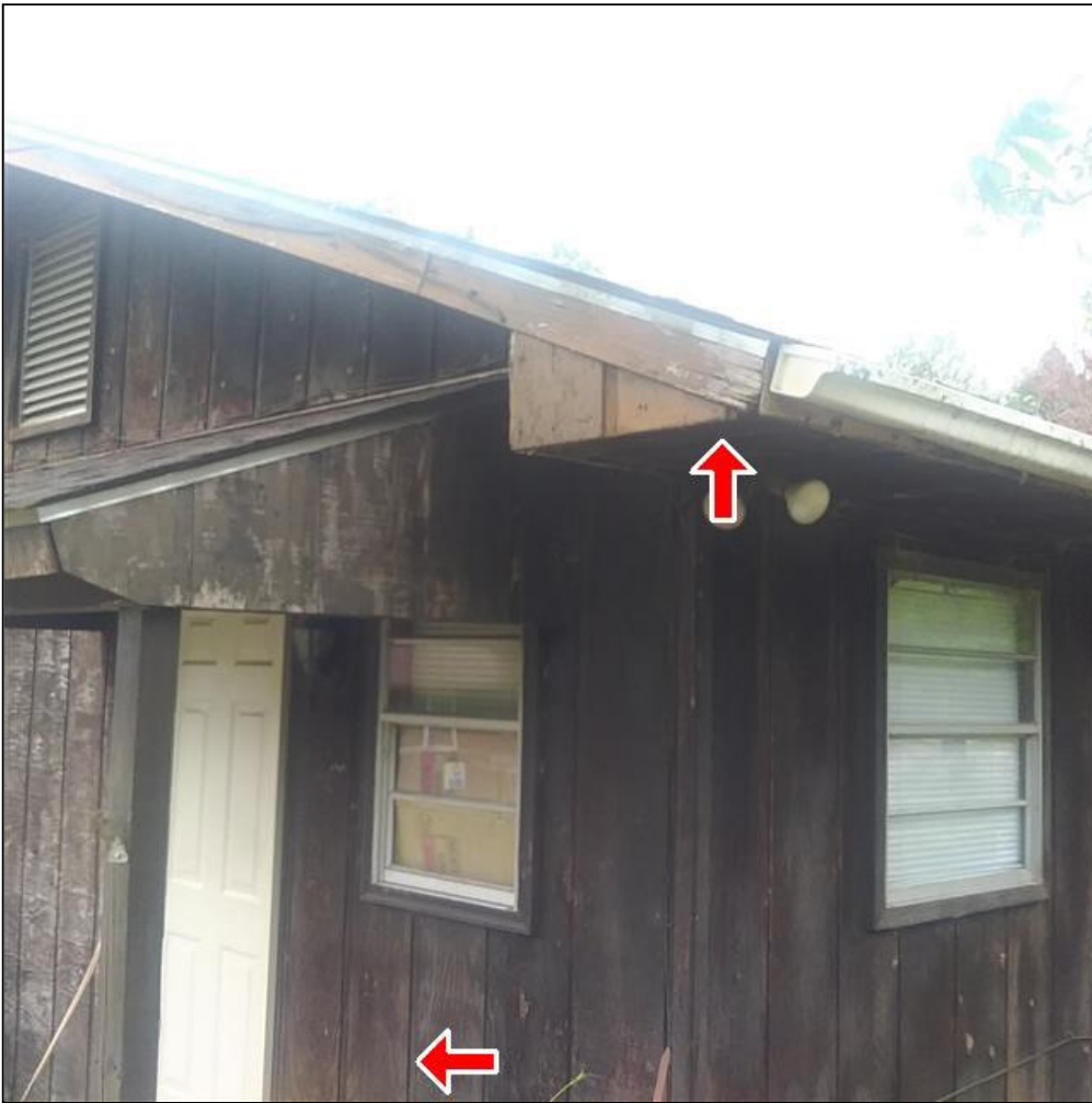
2.0 Item 3(Picture) Exterior wall siding, trim, and fascia on Cottage needs to be painted or stained to prevent wood rot.
