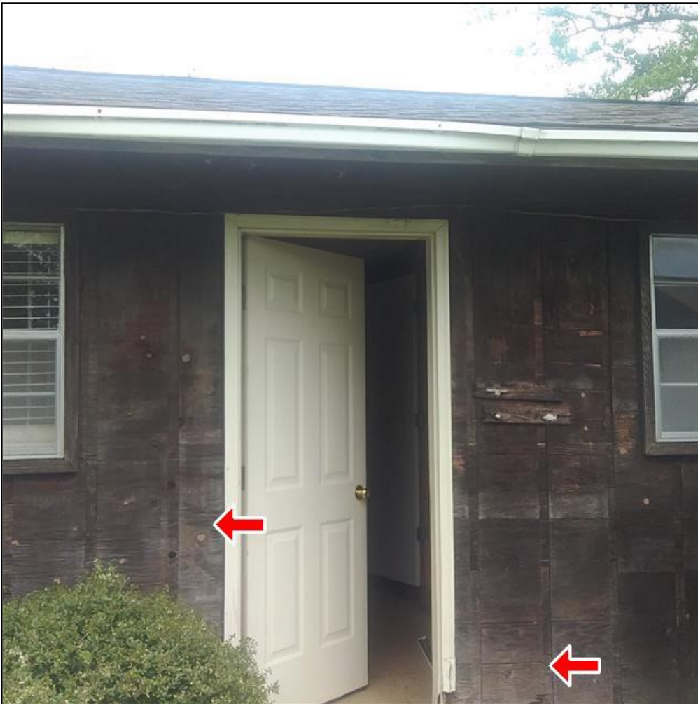
2.0 Item 2(Picture) Exterior wall siding, trim, and fascia on Cottage needs to be painted or stained to prevent wood rot.
