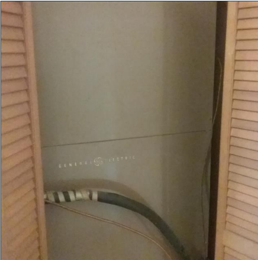
8.0 Item 3(Picture) The HVAC system serving the middle portion of home is at end of its expected service life, and will need to be replaced in the near future.
