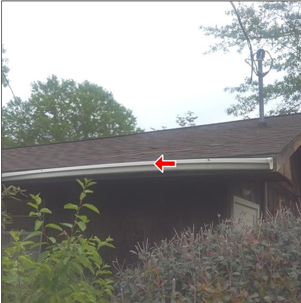
1.0 Item 2(Picture) Cottage roof gutter needs to be straightened or replaced.
