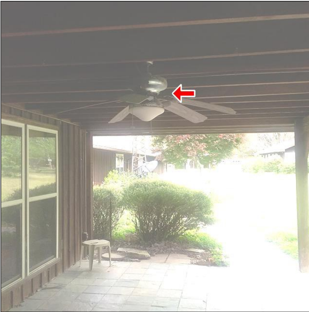
7.3 Item 1(Picture) The ceiling fan on the back needs to be replafed, as it has paint peeling off motor housing, and blades are drooping.
