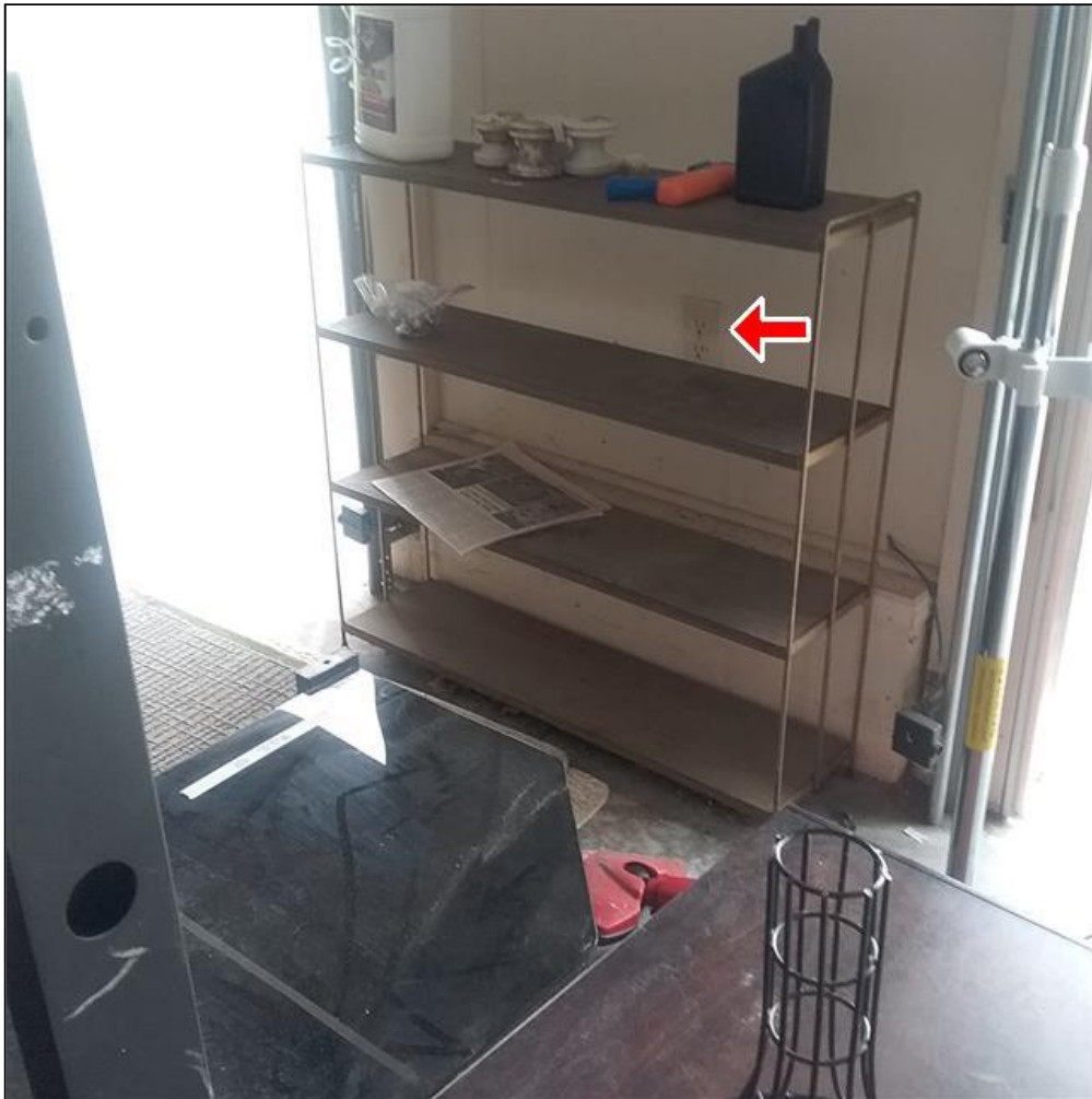
7.5 Item 4(Picture) Receptacle needs to be changed to GFCI type receptacle.
