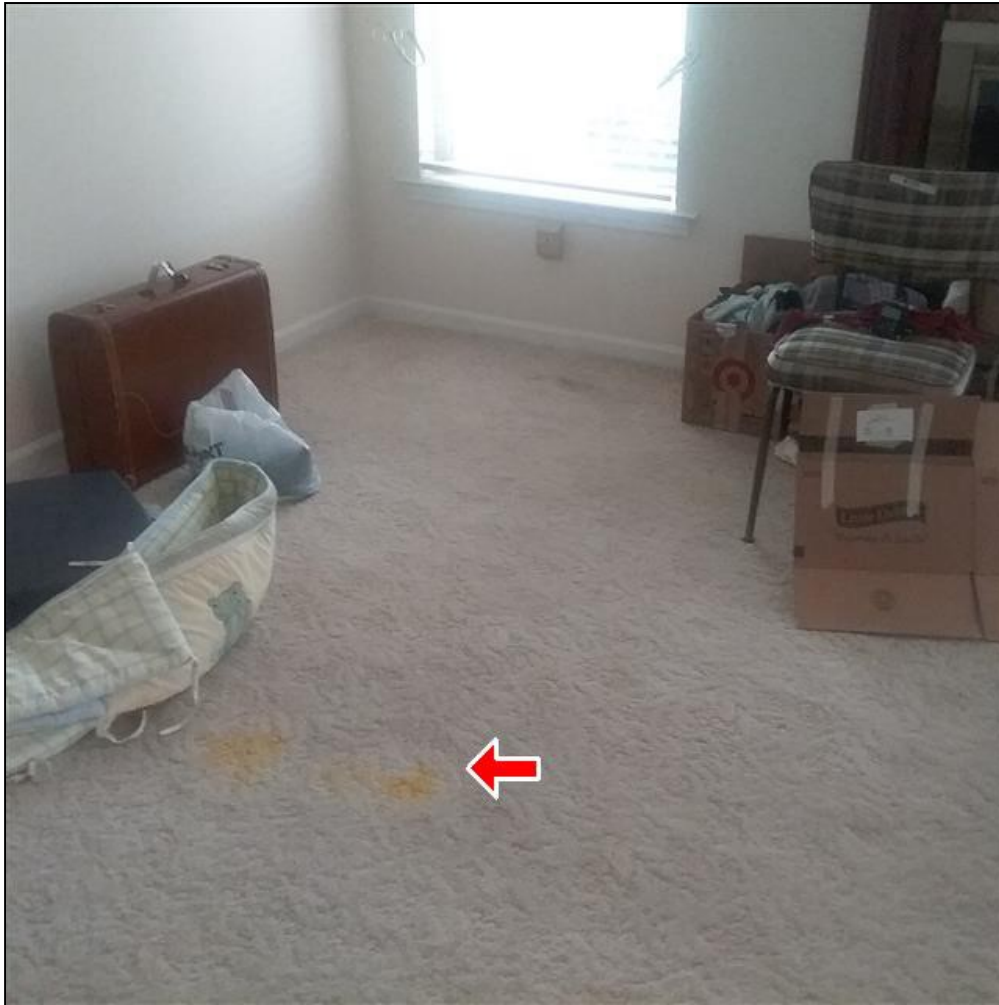
4.2 Item 1(Picture) Front right bedroom carpet needs to be replaced (2) The carpet in Cottage needs to be replaced.
