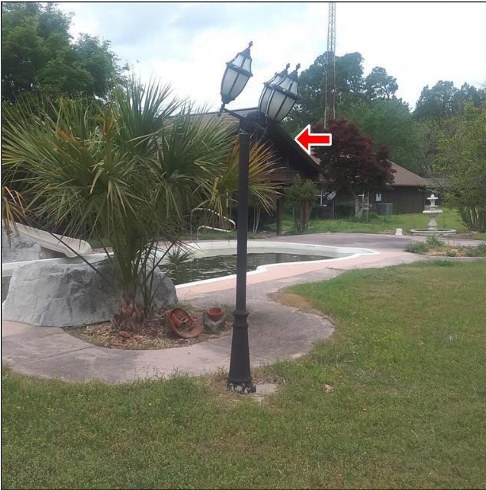
7.3 Item 4(Picture) The exterior post lamp needs repair.
