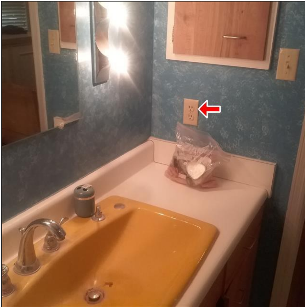
7.5 Item 1(Picture) Receptacle needs to be changed to GFCI type receptacle.
