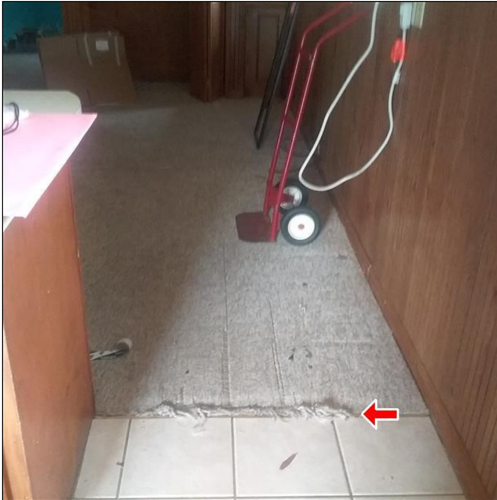
4.2 Item 3(Picture) The carpet in Cottage needs to be replaced.
