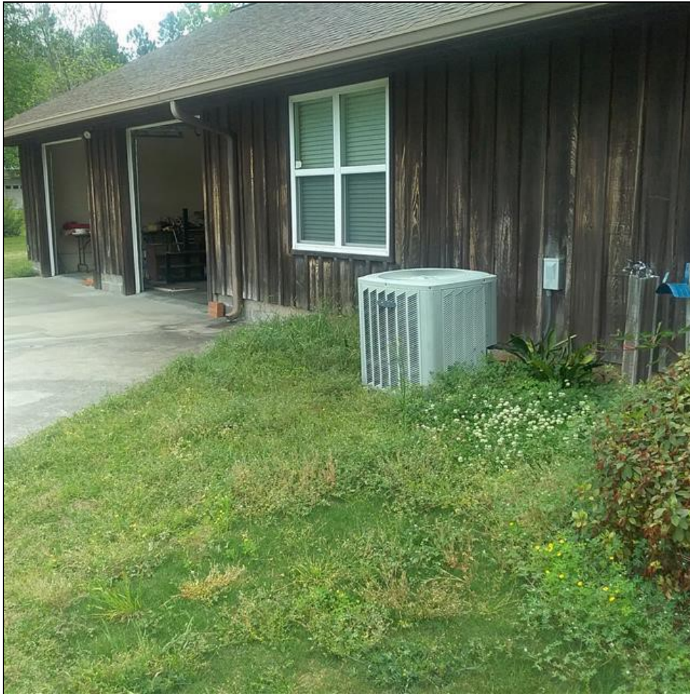
8.8 Item 2(Picture) The HVAC system serving the middle portion of home is at end of its expected service life, and will need to be replaced in the near future.
