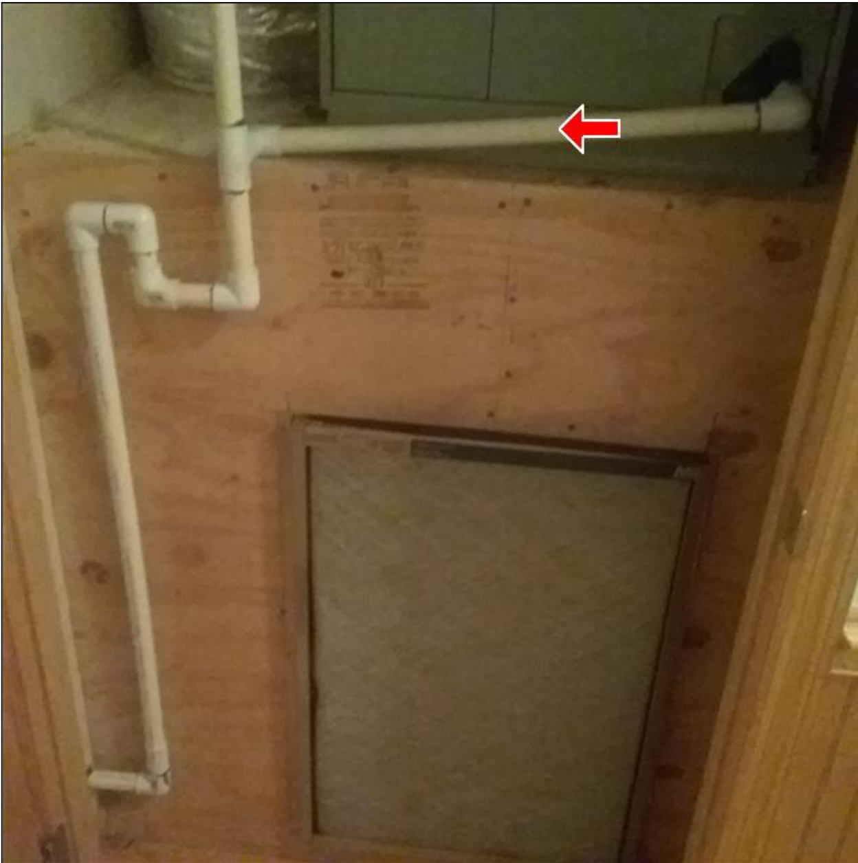
8.2 Item 1(Picture) All HVAC air handlers need to have condensate water shut off sensors installed on the primary drains.
