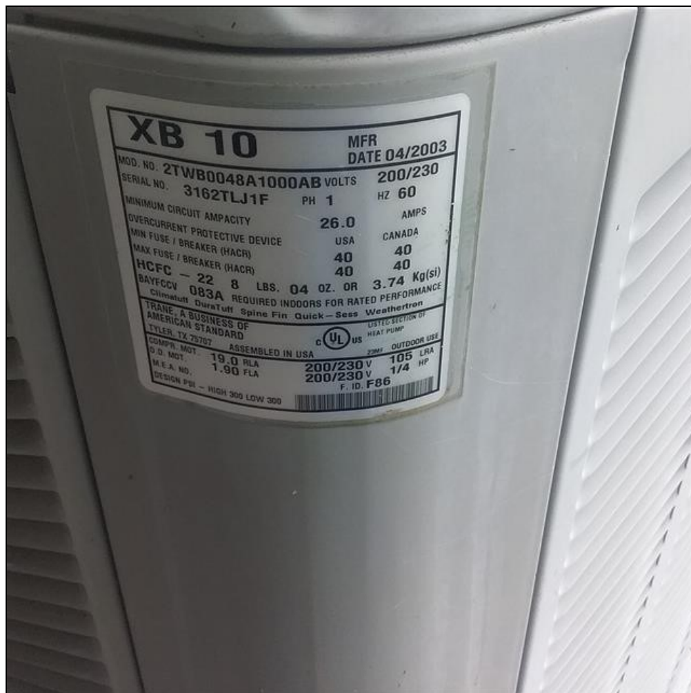
8.8 Item 3(Picture) The HVAC system serving the middle portion of home is at end of its expected service life, and will need to be replaced in the near future.
