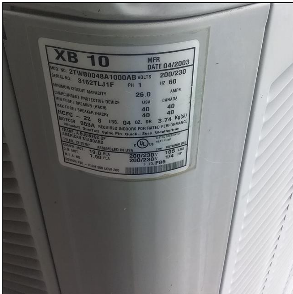
8.0 Item 2(Picture) The HVAC system serving the middle portion of home is at end of its expected service life, and will need to be replaced in the near future.
