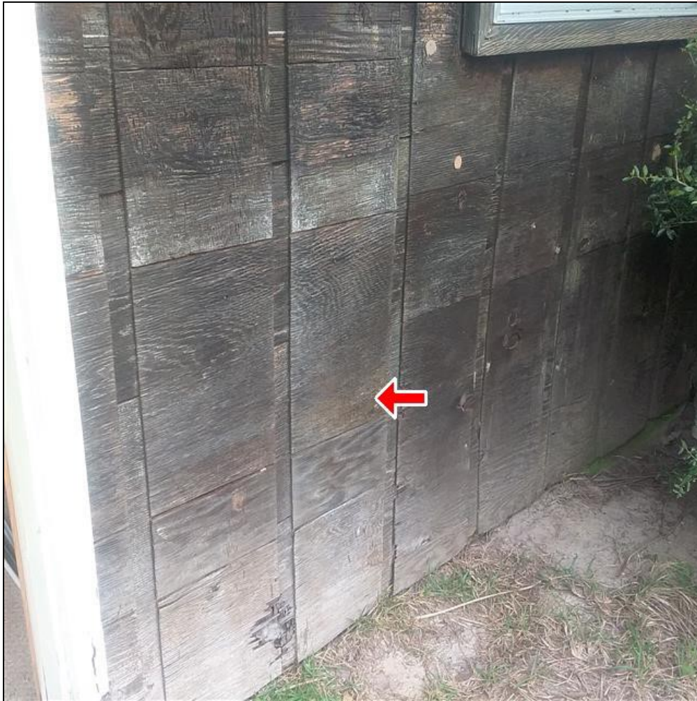
2.0 Item 1(Picture) Exterior wall siding, trim, and fascia on Cottage needs to be painted or stained to prevent wood rot.
