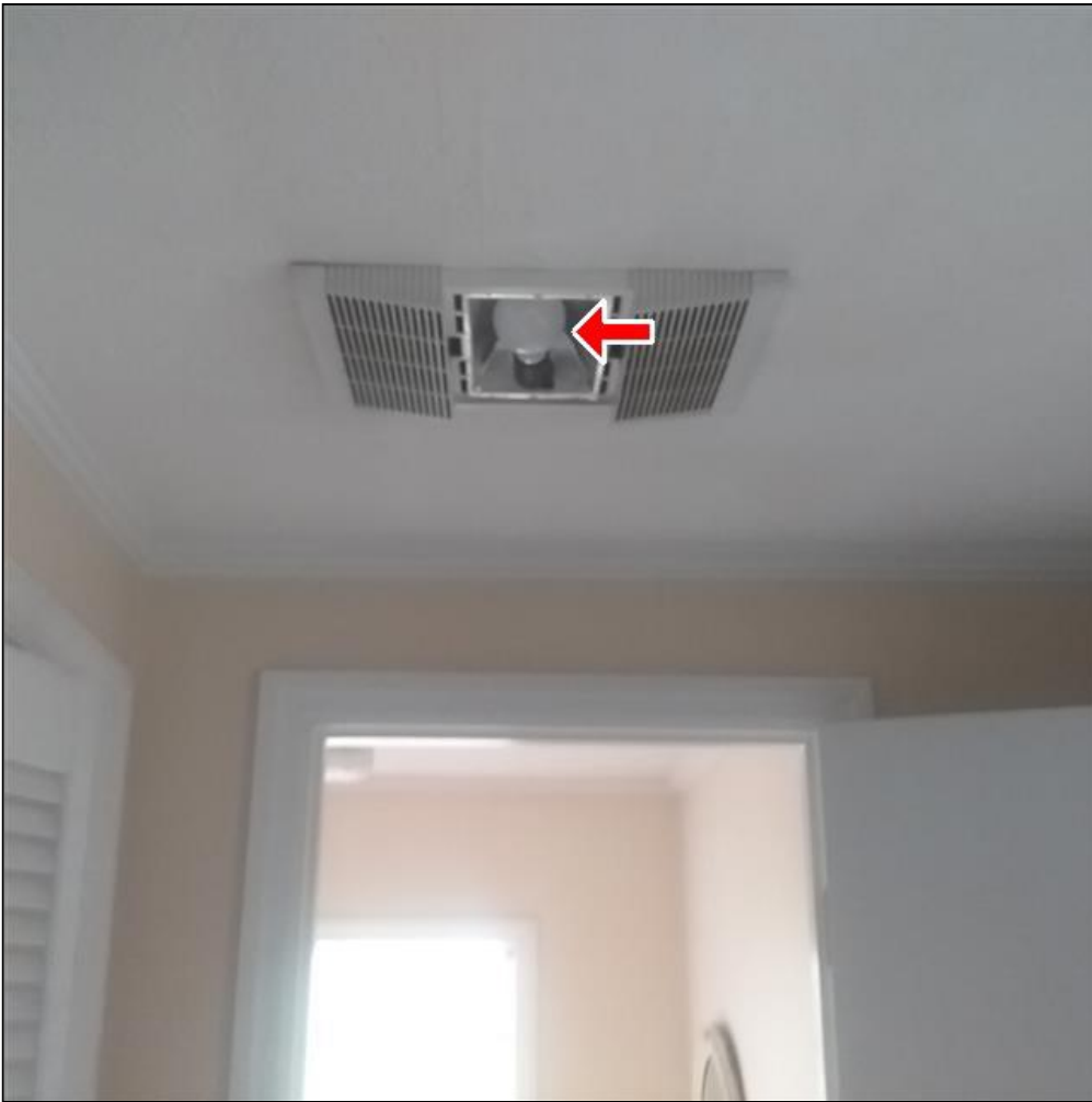
7.3 Item 3(Picture) Light needs cover in bathroom.
