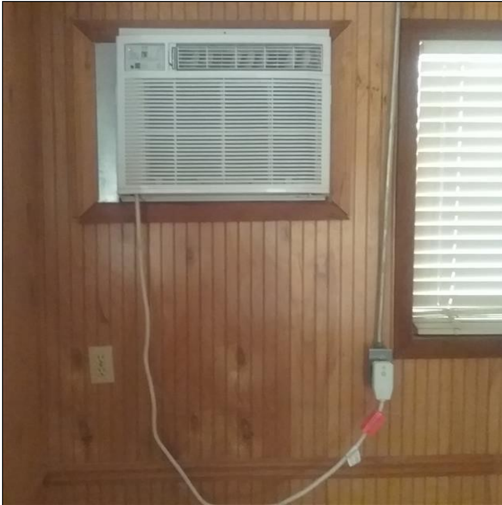
8.8 Item 1(Picture) Window AC unit in front of cottage not functioning when tested.
