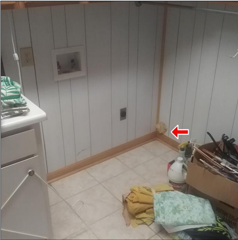
9.4 Item 2(Picture) There is no dryer vent stub kit installed.
