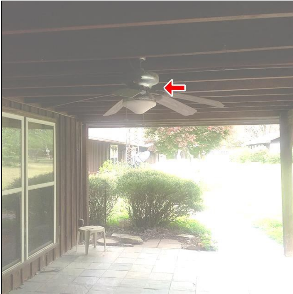
7.3 Item 1(Picture) The ceiling fan on the back needs to be replafed, as it has paint peeling off motor housing, and blades are drooping.
