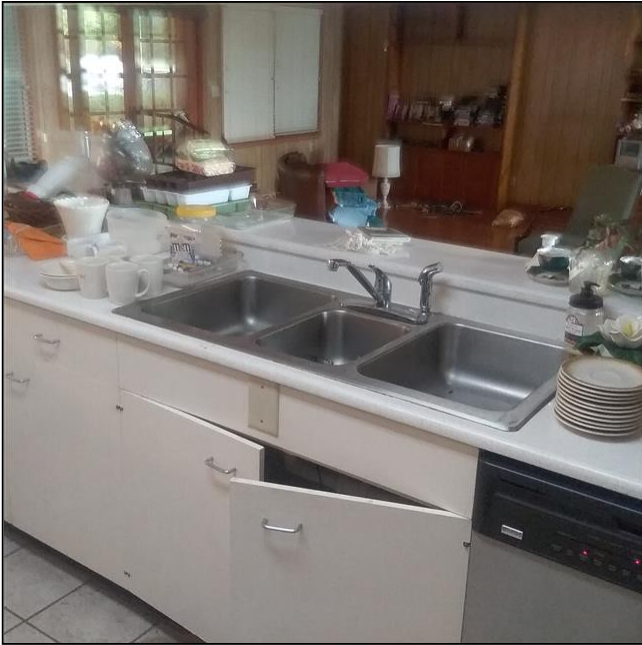
6.1 Item 1(Picture) The hot water side of kitchen faucet did not function when tested.
