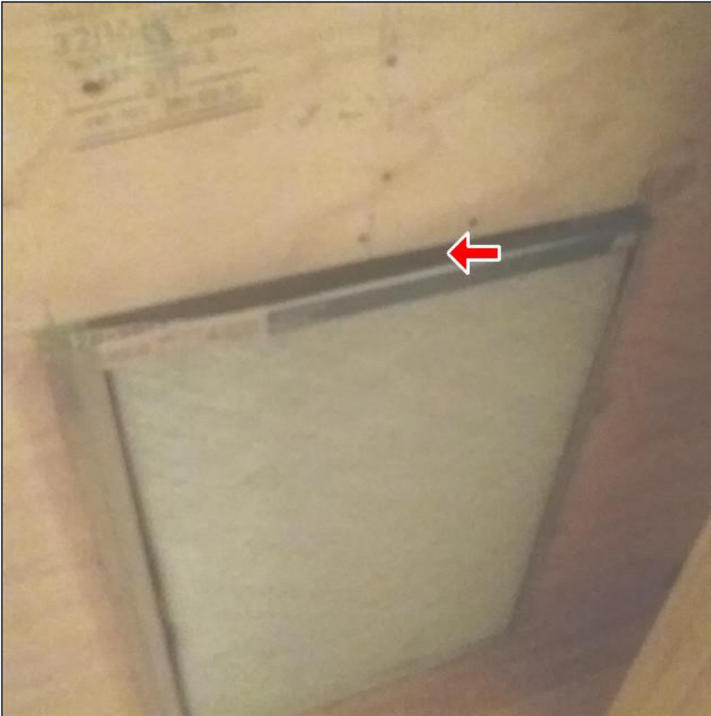
8.3 Item 1(Picture) Air is bypassing the filter at top on the HVAC system for left side of home. Filter needs a retainer to keep flat to wood box.
