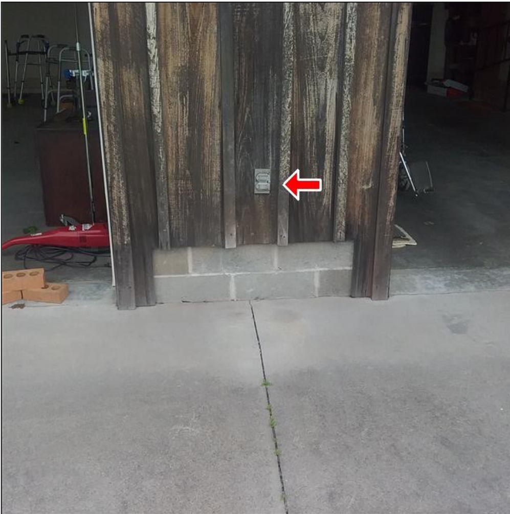
7.5 Item 3(Picture) Receptacle needs to be changed to GFCI type receptacle.
