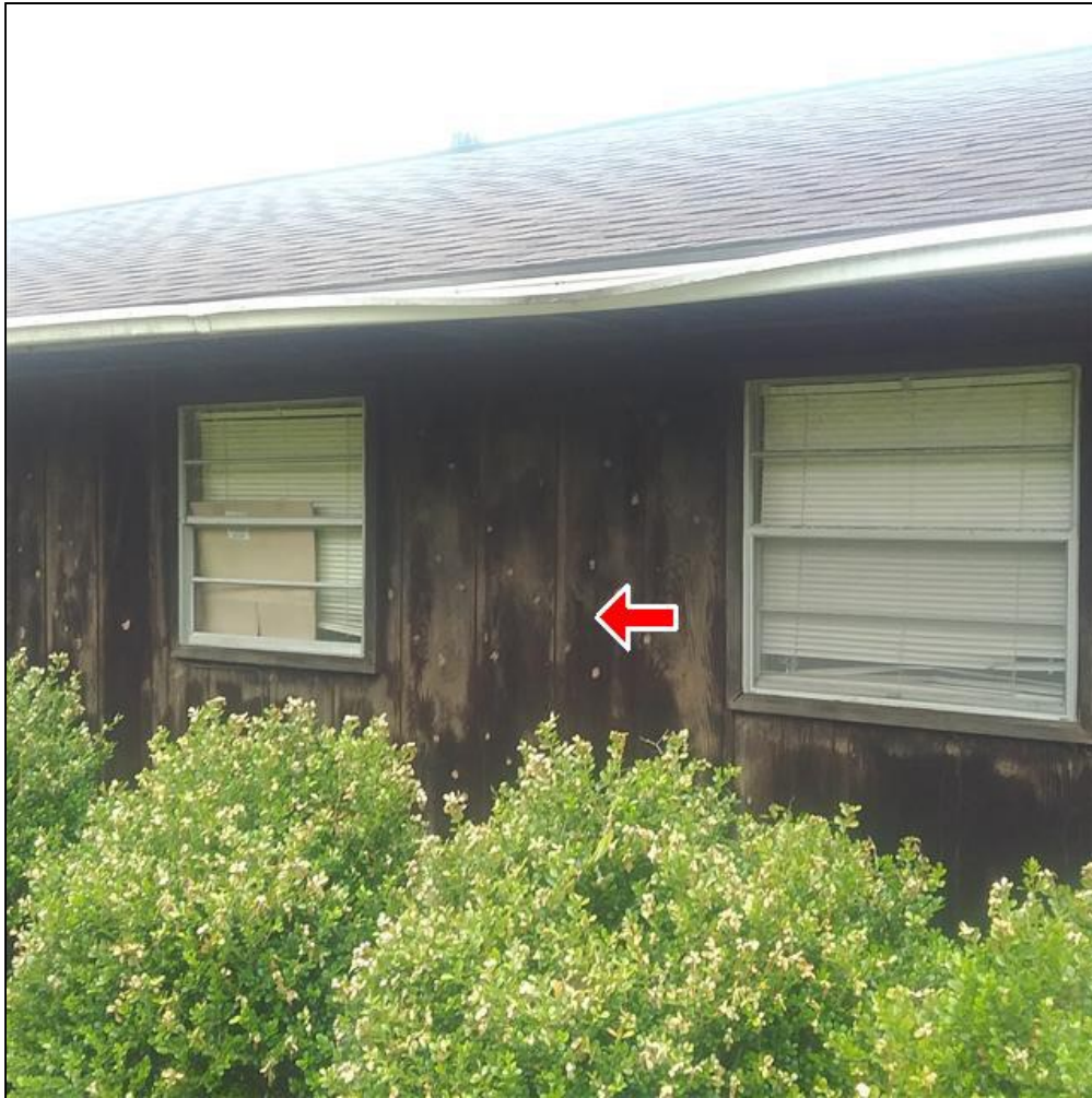
2.0 Item 4(Picture) Exterior wall siding, trim, and fascia on Cottage needs to be painted or stained to prevent wood rot.
