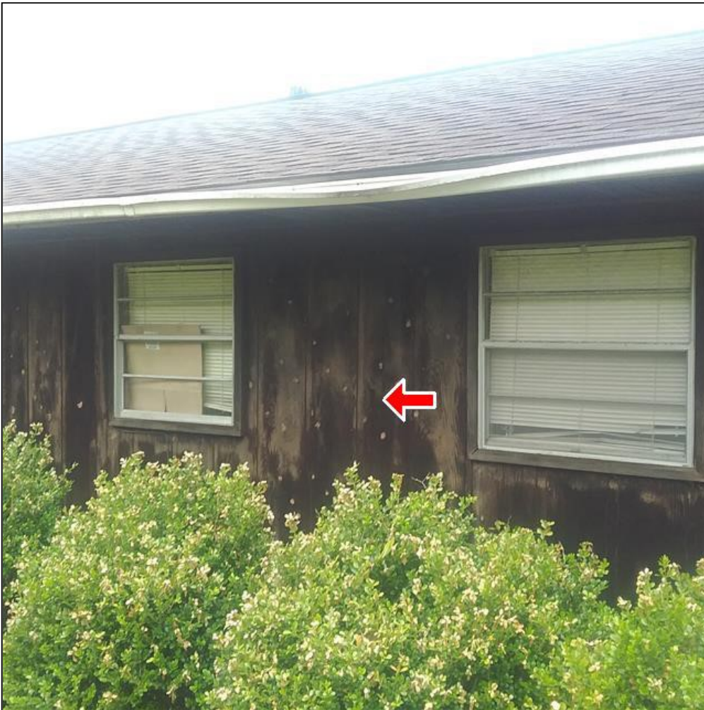
2.0 Item 4(Picture) Exterior wall siding, trim, and fascia on Cottage needs to be painted or stained to prevent wood rot.
