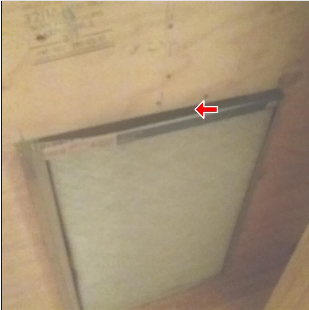
8.3 Item 1(Picture) Air is bypassing the filter at top on the HVAC system for left side of home. Filter needs a retainer to keep flat to wood box.
