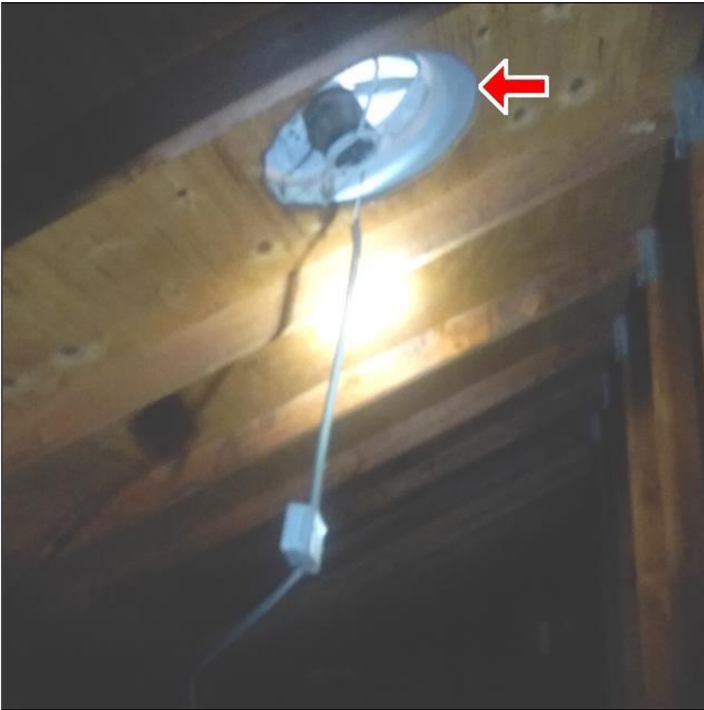
9.5 Item 1(Picture) Both roof attic power ventilator motors are bad, and need to be replaced.
