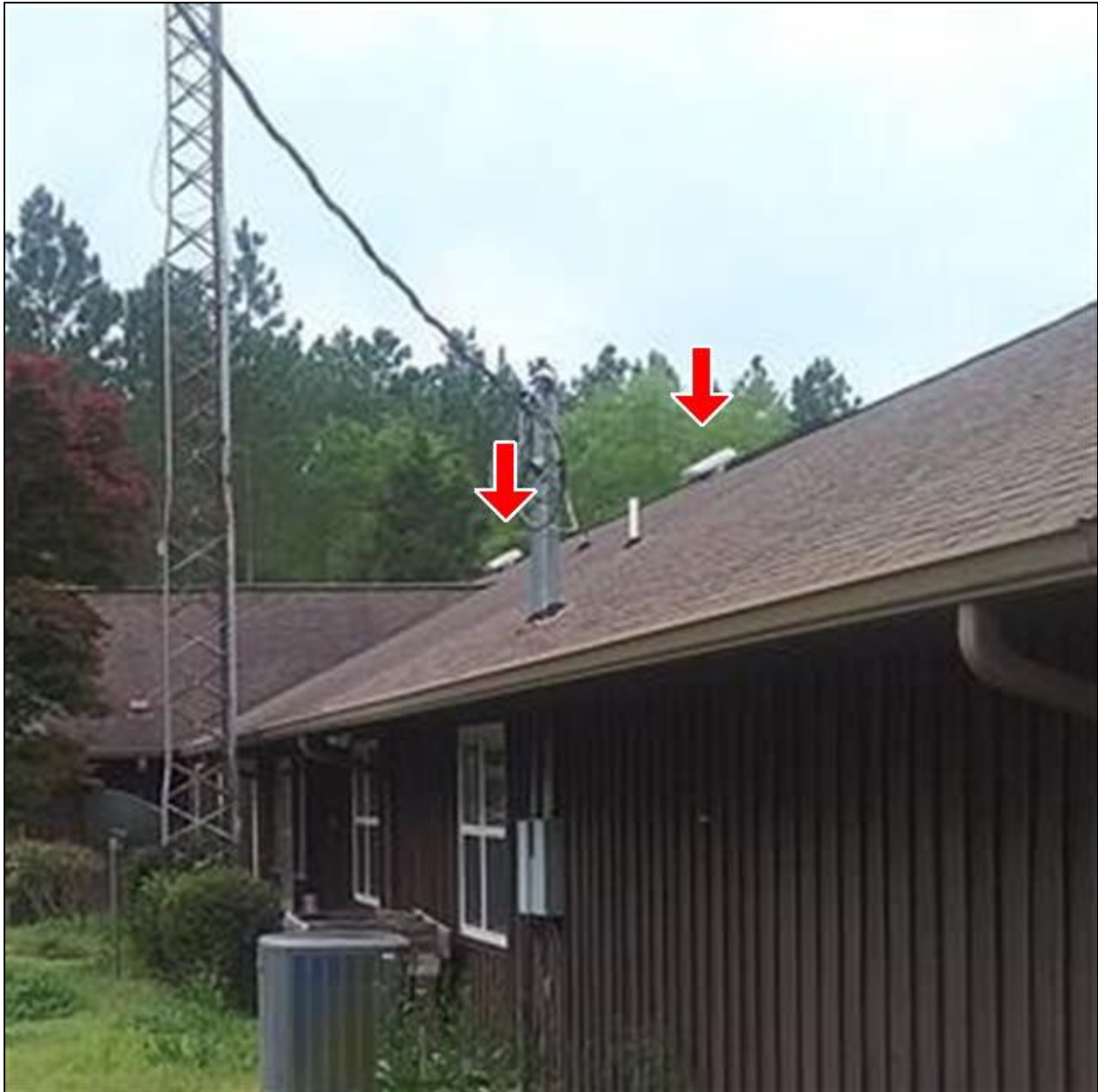
9.5 Item 2(Picture) Both roof attic power ventilator motors are bad, and need to be replaced.
