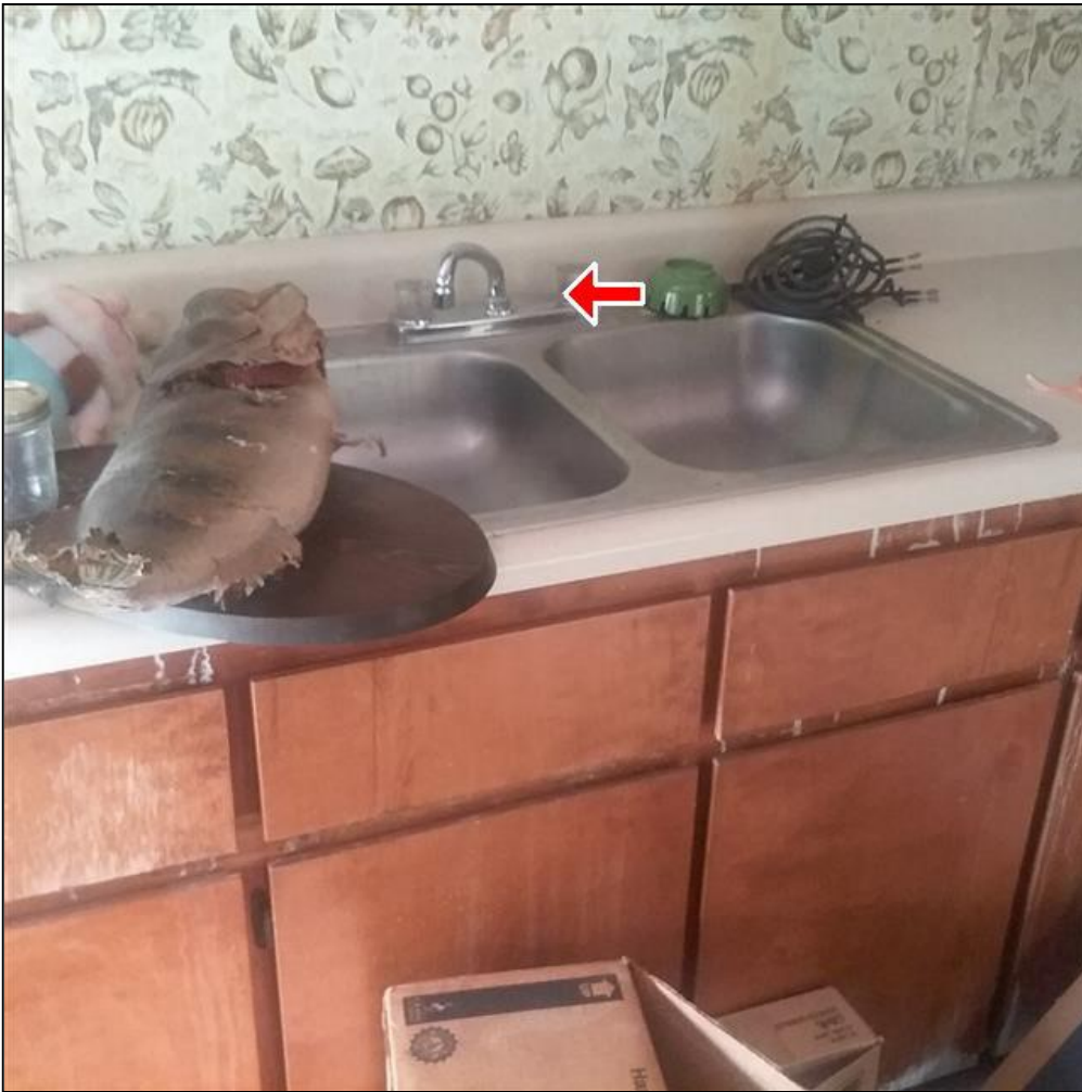
6.1 Item 2(Picture) The hot water side of Cottage kitchen faucet did not function when tested..
