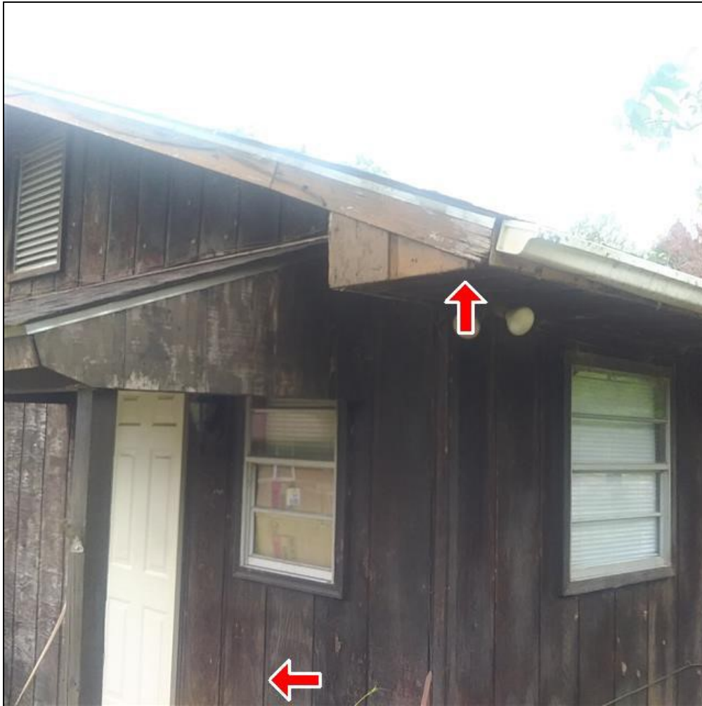
2.0 Item 3(Picture) Exterior wall siding, trim, and fascia on Cottage needs to be painted or stained to prevent wood rot.
