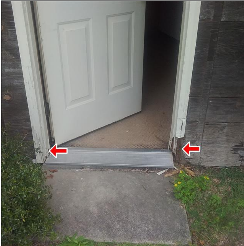
2.1 Item 1(Picture) The wood door trim has water damage needing to be repaired, or replaced.
