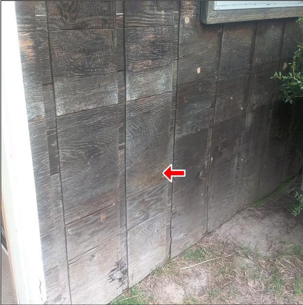
2.0 Item 1(Picture) Exterior wall siding, trim, and fascia on Cottage needs to be painted or stained to prevent wood rot.
