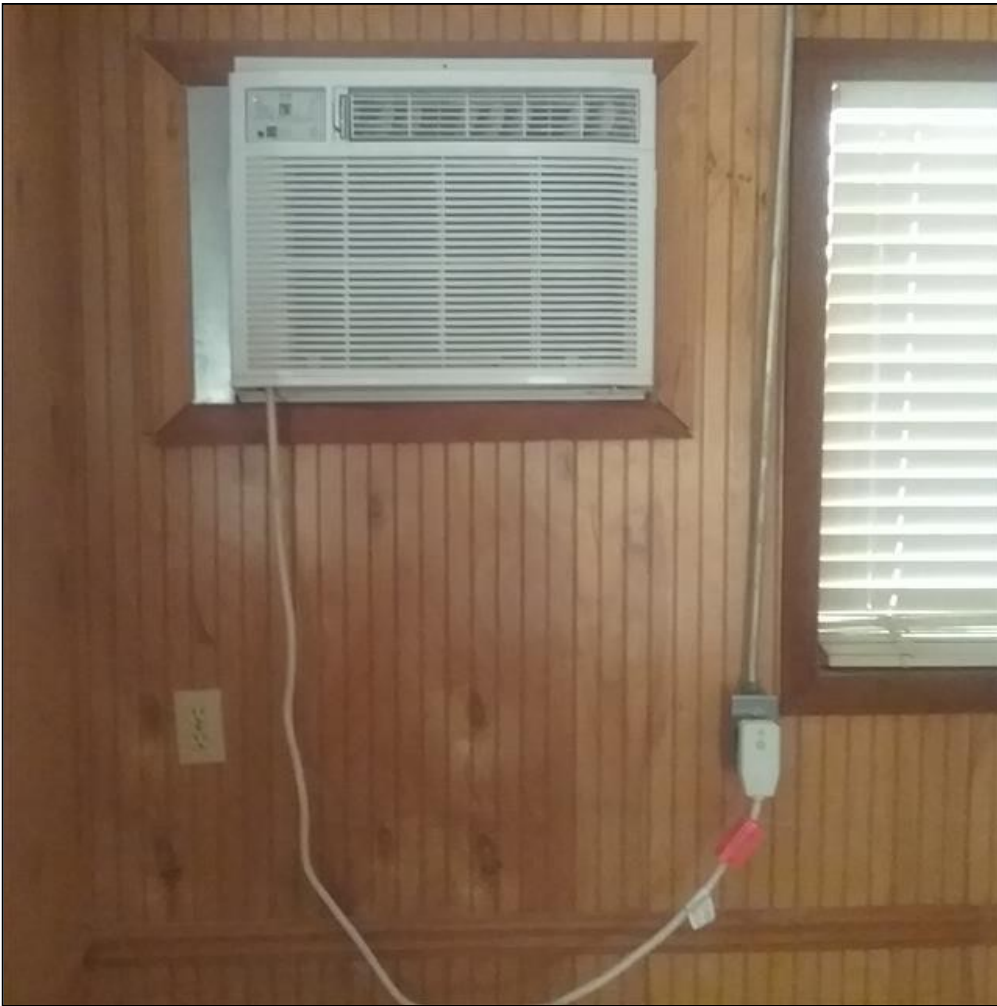
8.8 Item 1(Picture) Window AC unit in front of cottage not functioning when tested.
