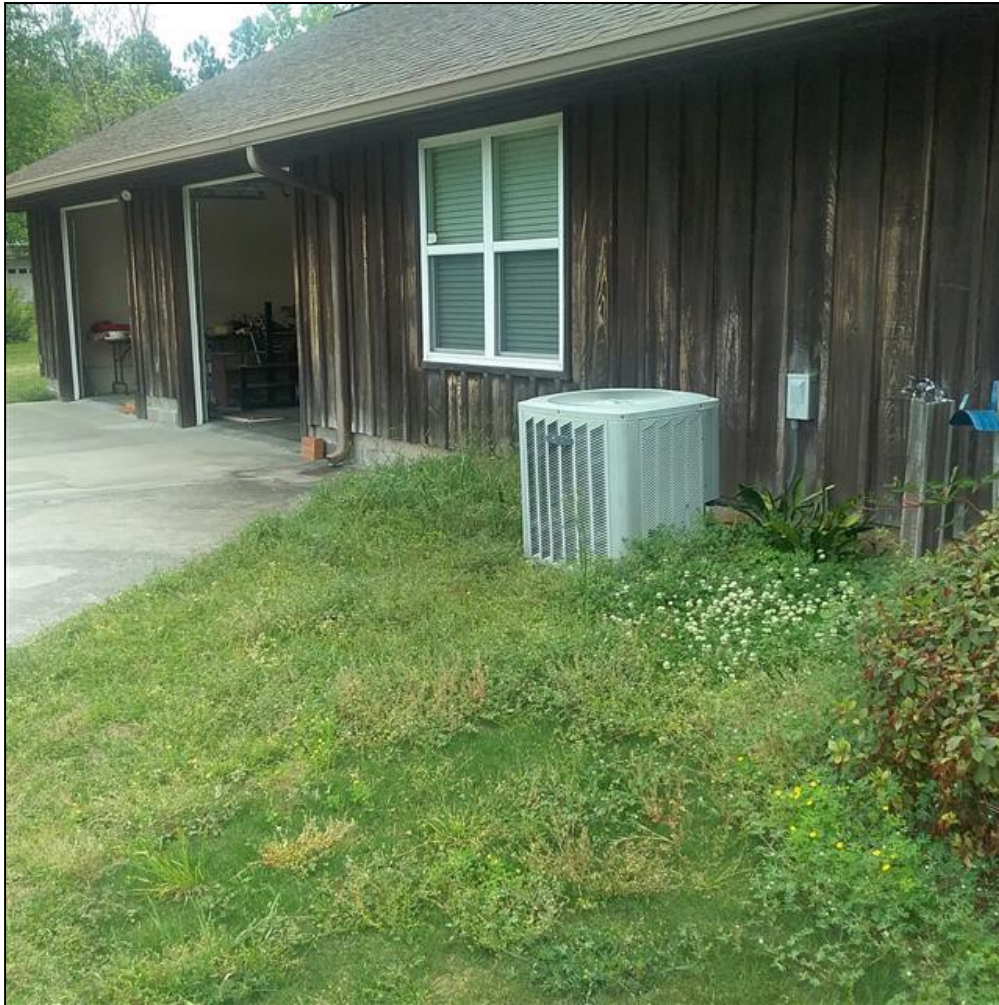
8.0 Item 1(Picture) The HVAC system serving the middle portion of home is at end of its expected service life, and will need to be replaced in the near future.
