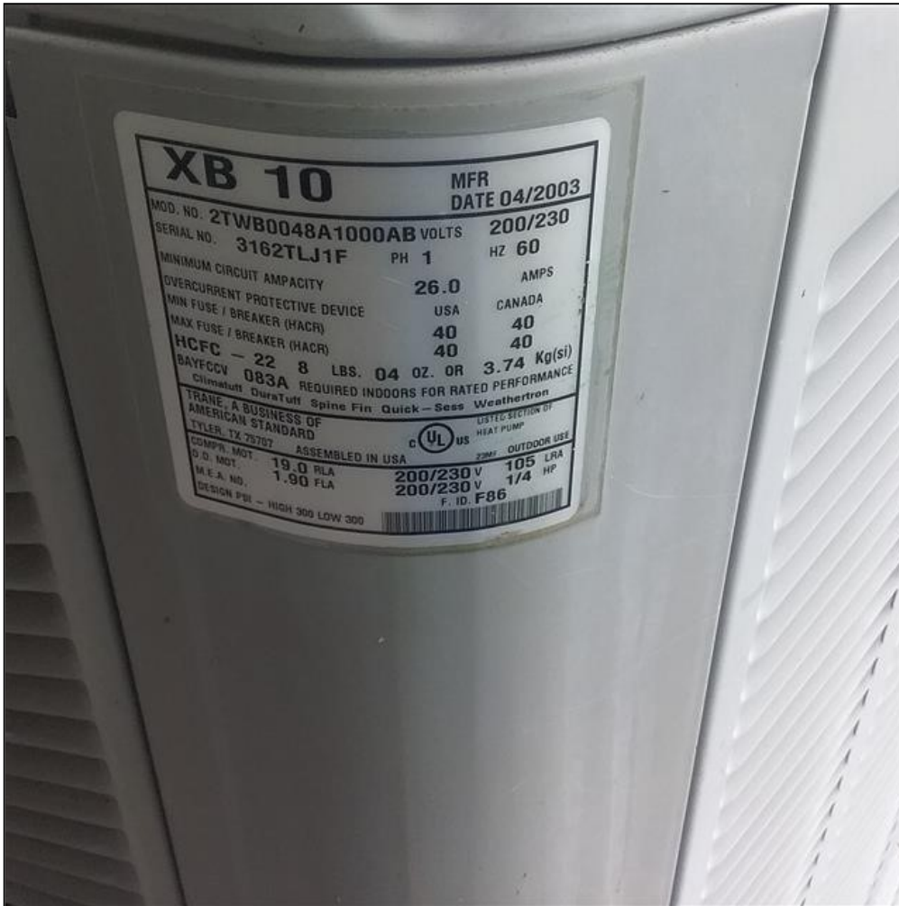
8.0 Item 2(Picture) The HVAC system serving the middle portion of home is at end of its expected service life, and will need to be replaced in the near future.
